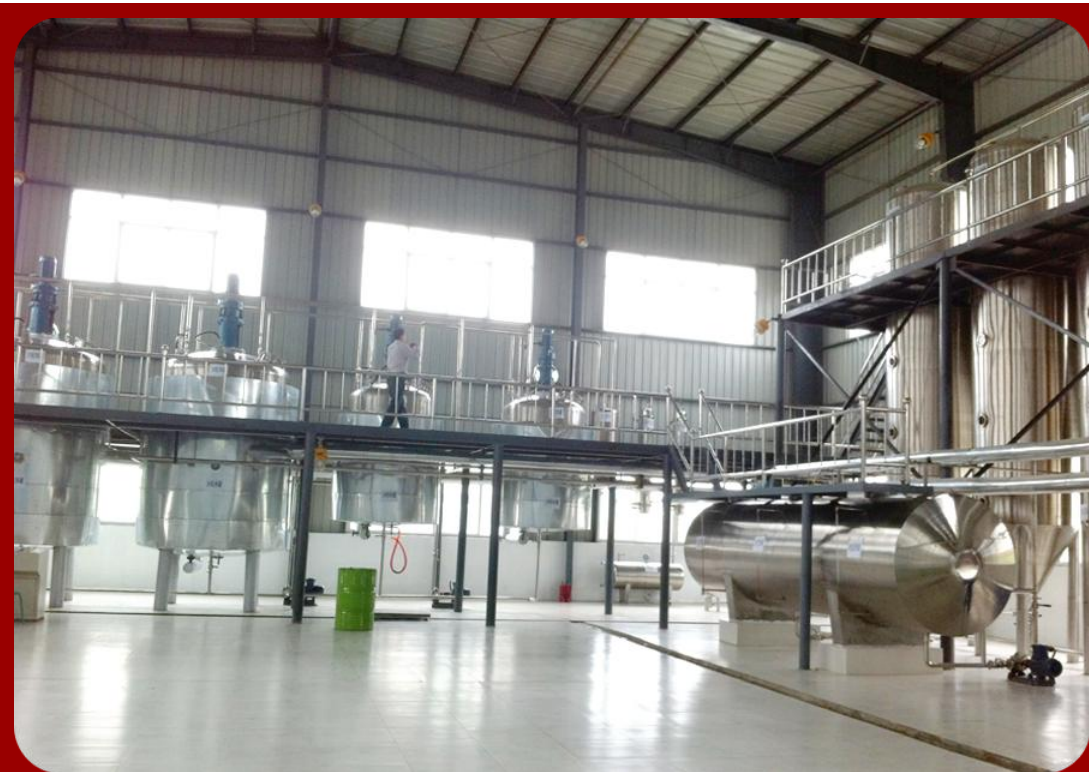
精制设备 Refining equipment
