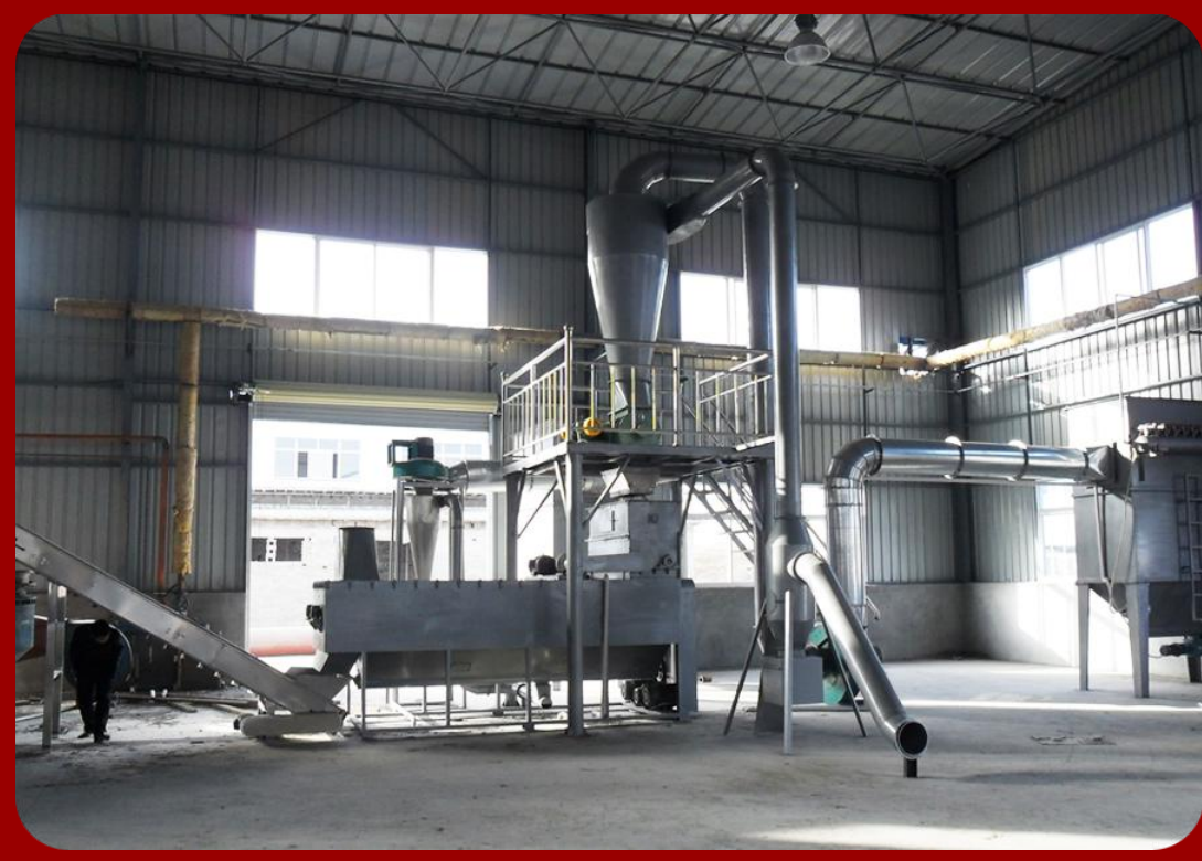
去籽机除尘设备 Dedusting equipment
